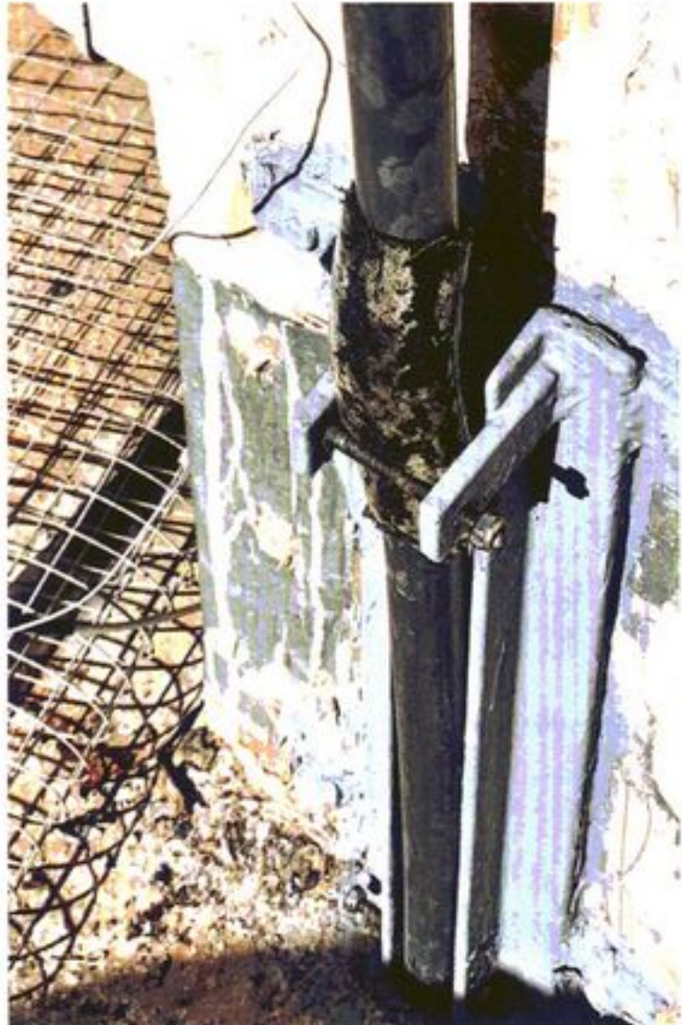
Fixed to the wall with a flexible section of pipe, showing the wire mesh 'earth
